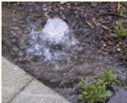
Repair broken sprinkler heads like this one before you run an irrigation audit on your system.
