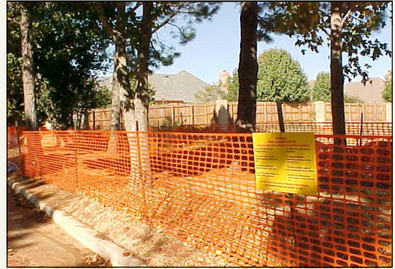
As of November 2007, the City of Southlake now requires that tree conservation plans and tree protection details be posted on all construction sites.
